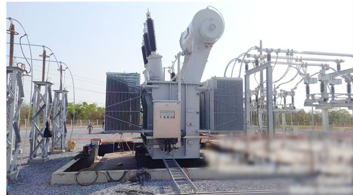
DIY self supply high voltage transformer
